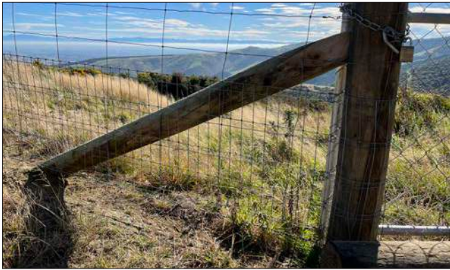
Equine mesh is being installed on the deer fence to deter feral pigs
